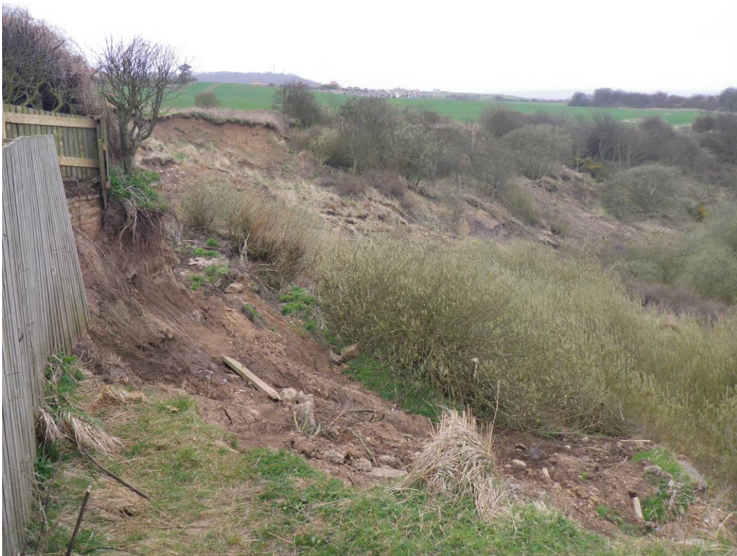
Plate 2 Slope failures on Cornelian Bay side of Knipe Point looking northwest
