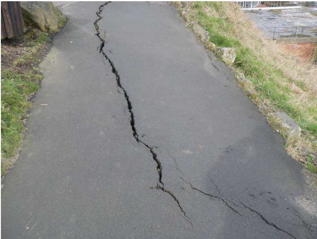
Plate 54 Scarborough South Cliff. Pavement cracks above the Clock Café (March. 2010)
