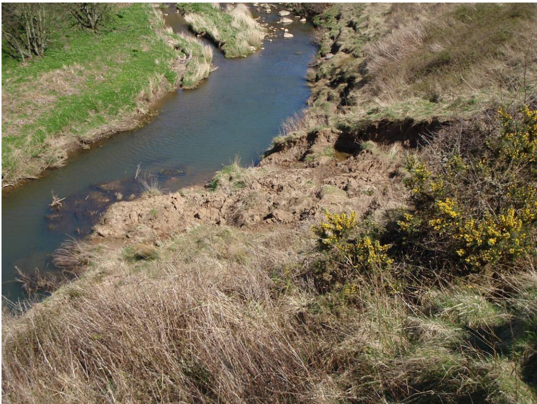
Plate 6 Slope failure along river's edge of Behavioural Unit I. (14 th April 2010)
