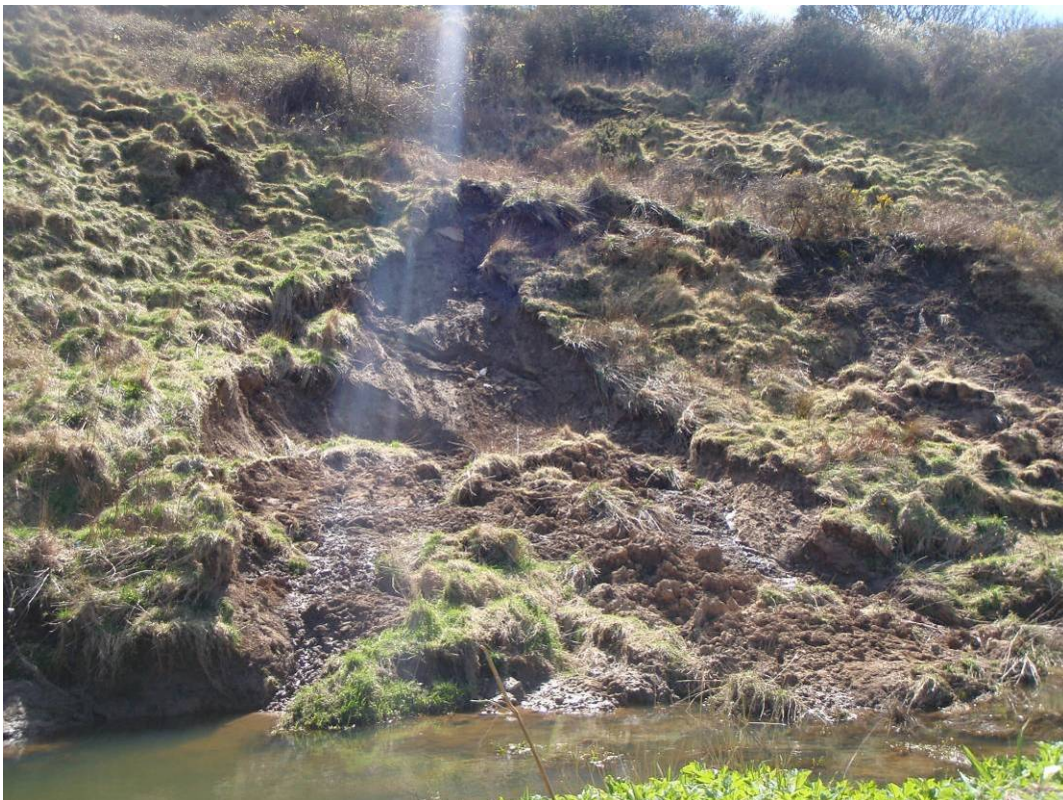
Plate 3 Slope failure along river's edge of Behavioural Unit I. (14 th April 2010)
