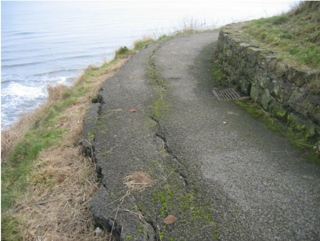
Plate 57 Footpath degradation around Holbeck Gardens.
